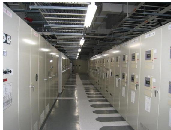
Extra high voltage power receiving panel
