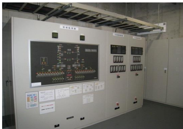
Extra high voltage power receiving monitoring and control system
