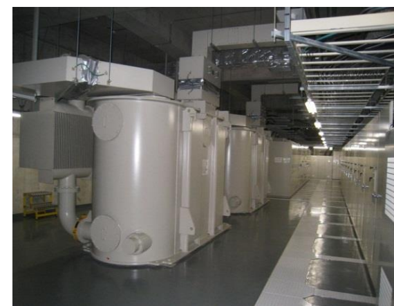
Extra high voltage power transformer
